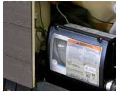
This allows access to spa components.
